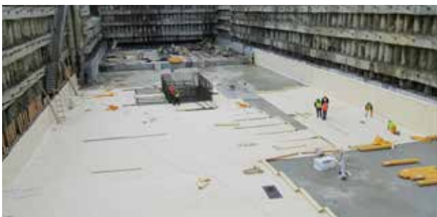
Vertical excavation wall, typically use for SikaProof® A under the raft and at the walls.
