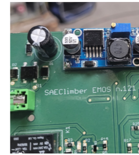
EMOS + 4.0 ELECTRONIC CARDS: This electronic devices included on the power panel, allows remote monitoring and balanced motors consumption.
