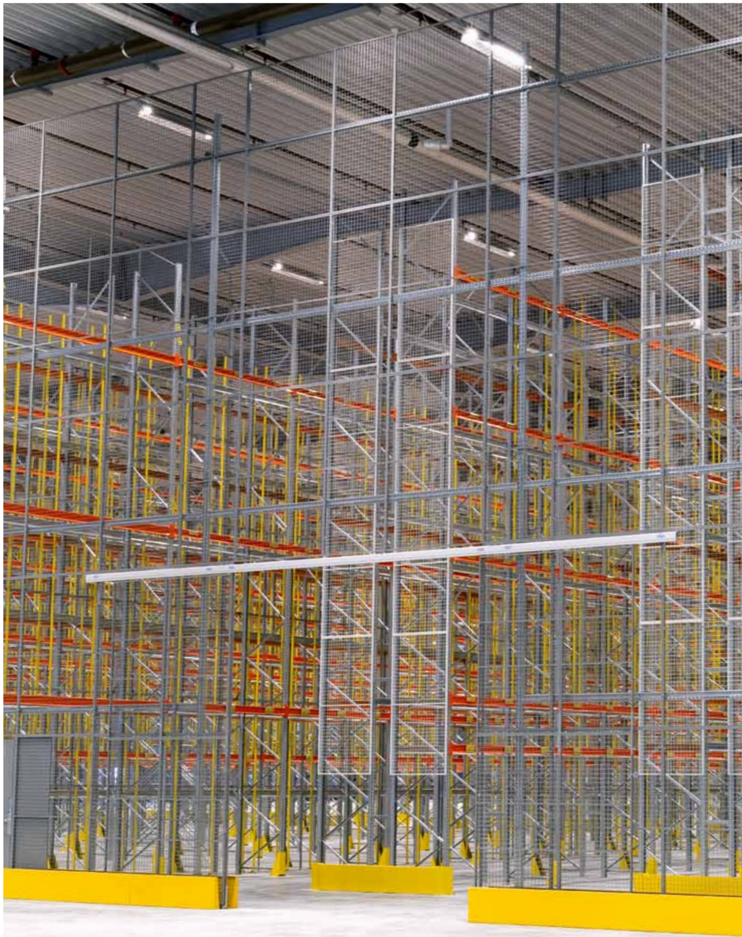
i The picture shows a secure storage installation using our Caelum system. The installation required an 11 metre high wall that was attached to the racking end frames. A double sliding door in a single rail was also installed for access.
